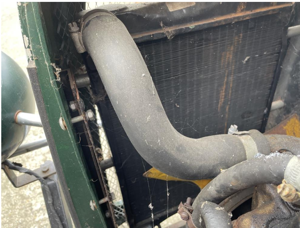
Original setup, not the best of installations or fixings.
